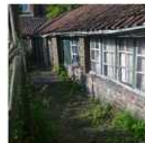
nagels in houten raamlat, roestig
